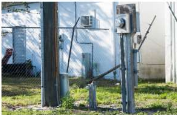
Image 11 – Timer and power connection for main street irrigation near 7 th Street. Main Street irrigation is not controlled by County. Question 6 conduit stub-ups and communication cable from pole
